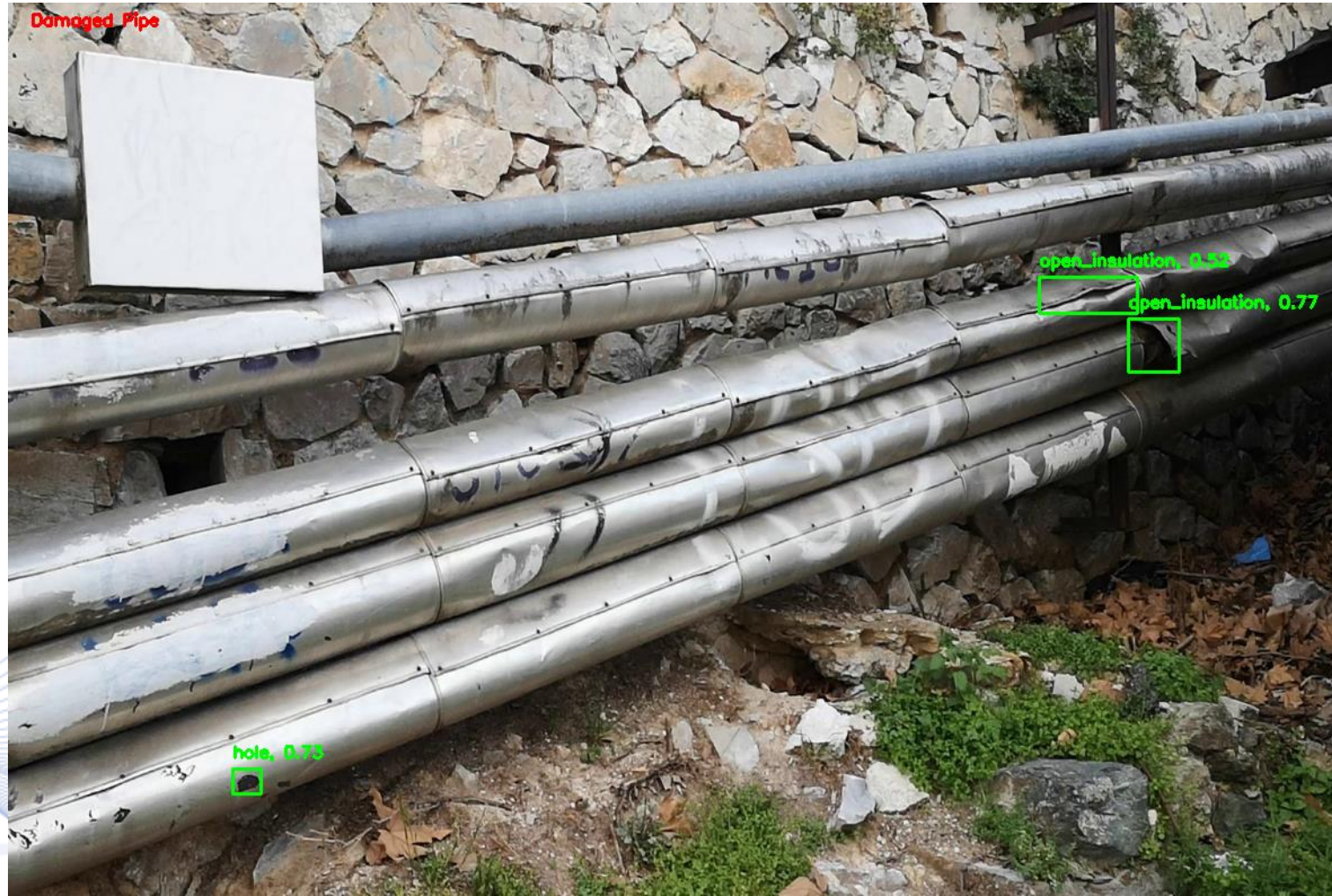
Pipe defect detection.
